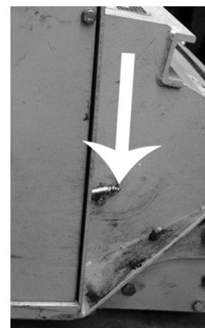
Rotor shaft greasing
